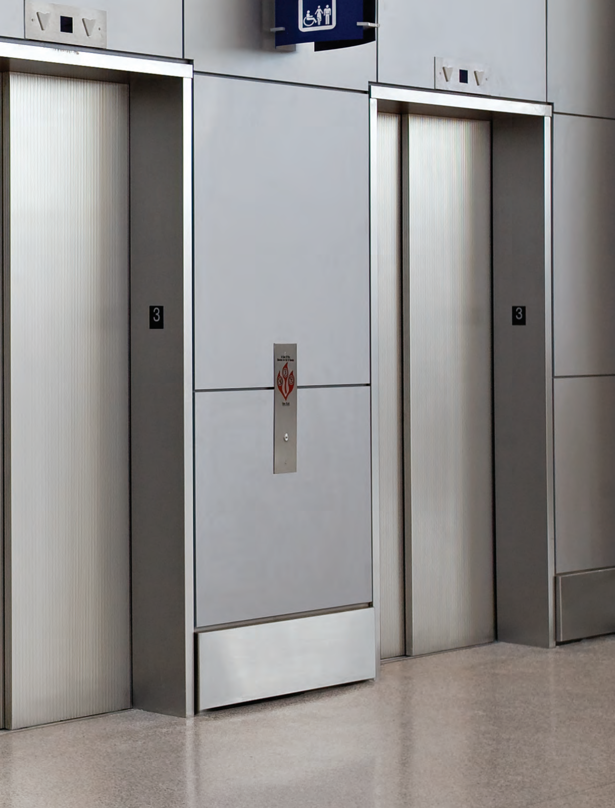
Stainless Steel Elevator Doors in Stainless Steel, Sandstone finish, Dallas Impression pattern. Indianapolis International Airport, Indianapolis, Indiana.
